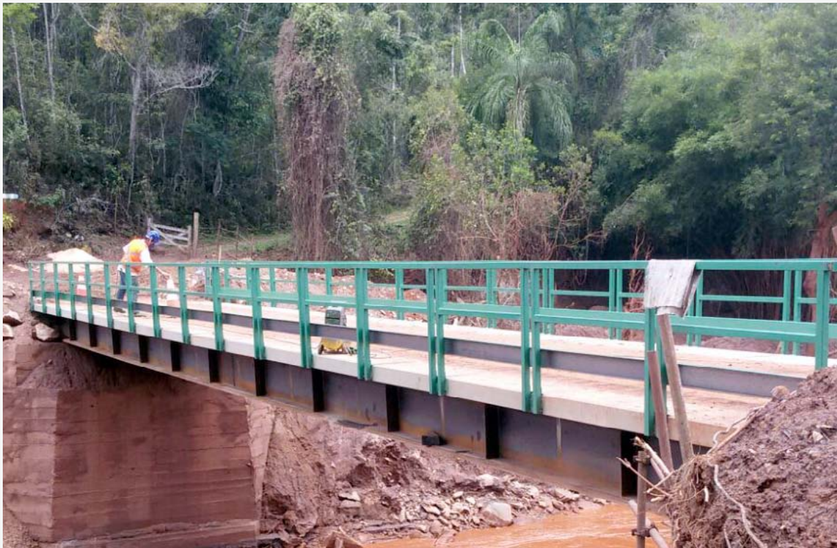
Bridge linking the districts of Aguas Claras and Monsenhor Horta is ready for use
