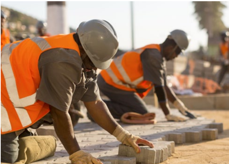
Alternatives for the use of the tailings are being studied and implemented by Samarco, such as the application of interlocking pavers in Barra Longa
